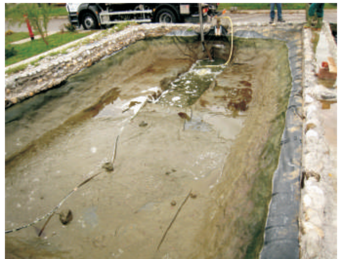
Untreated pond: Pond lining was covered with biofilm which was hard to remove even after scrubbing the lining.
