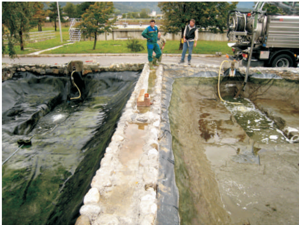
The untreated pond (right) contains a thick layer of biofilm even after cleaning.
